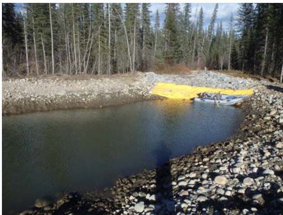
Plate 5. Looking downstream at the outlet of the downstream cell of Sediment Trap 3.
