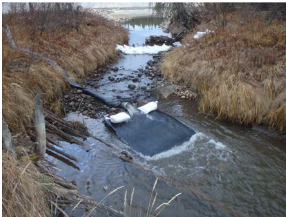
Plate 3. Looking upstream at the Sediment Trap 2B flow pump around discharge.
