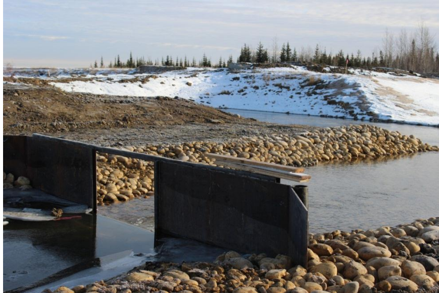
Main Tailings Pond Weir with Boards Removed and Clean Discharge
