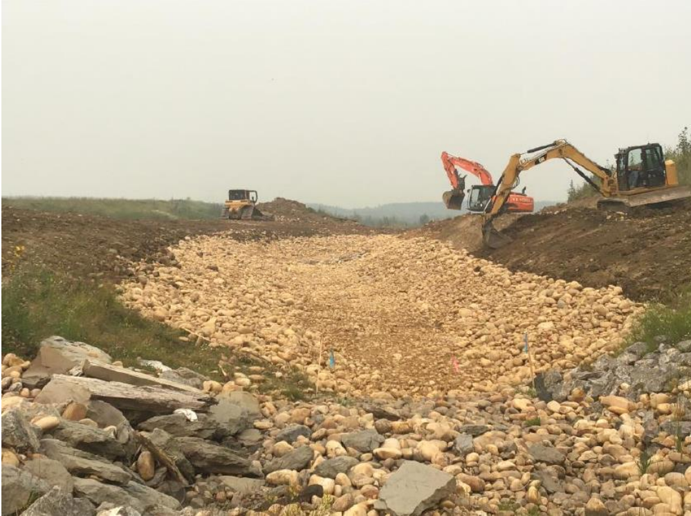
August 15, 2018: Looking downstream from 0+060 at channel shaping above the Class 1 rounded in preparation of topsoil placement and seeding/planting. Fines on the channel surface will be flushed using pumped water.
