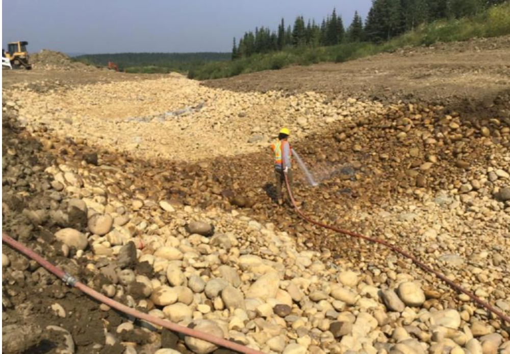
August 18, 2018: Looking downstream from 0+080 at APC-1 flushing using hose connected to trash pump.
