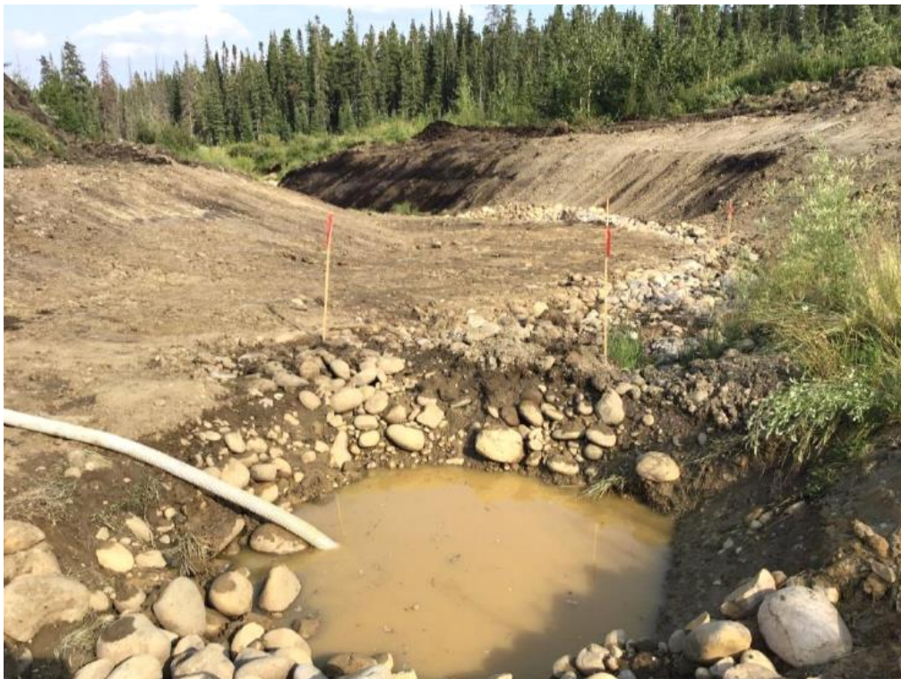
August 19, 2018: Looking downstream from 0+360 at constructed floodplain excavation for natural channel design. The natural channel design will start at about 0+350. This starting location will provide an extra 50 m of natural channel compared to design (sump in foreground; water from sump is being pumped to well vegetated areas away from the natural watercourse).
